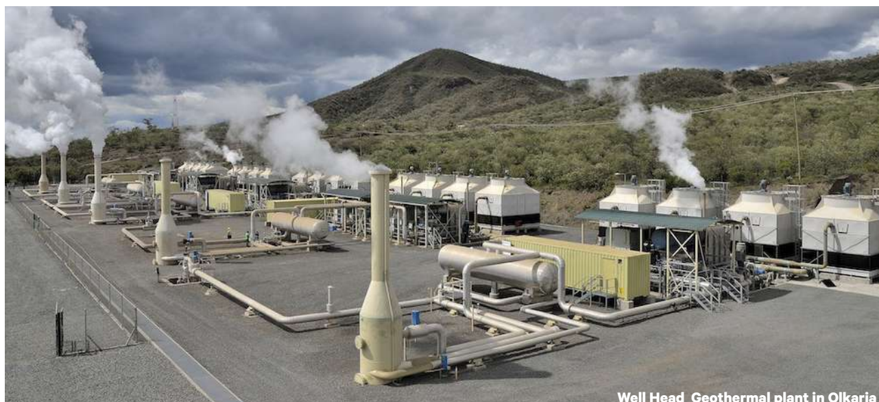
Well Head Geothermal plant in Olkaria
