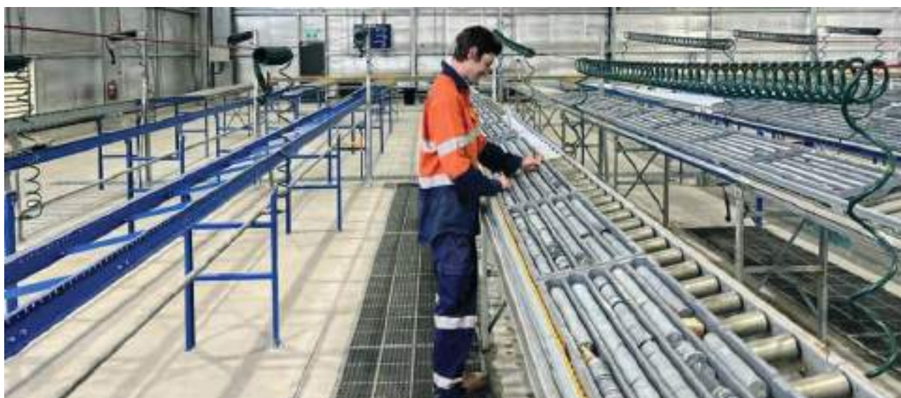
Mineral certification laboratory at Madini House being installed with specialised laboratory equipment
