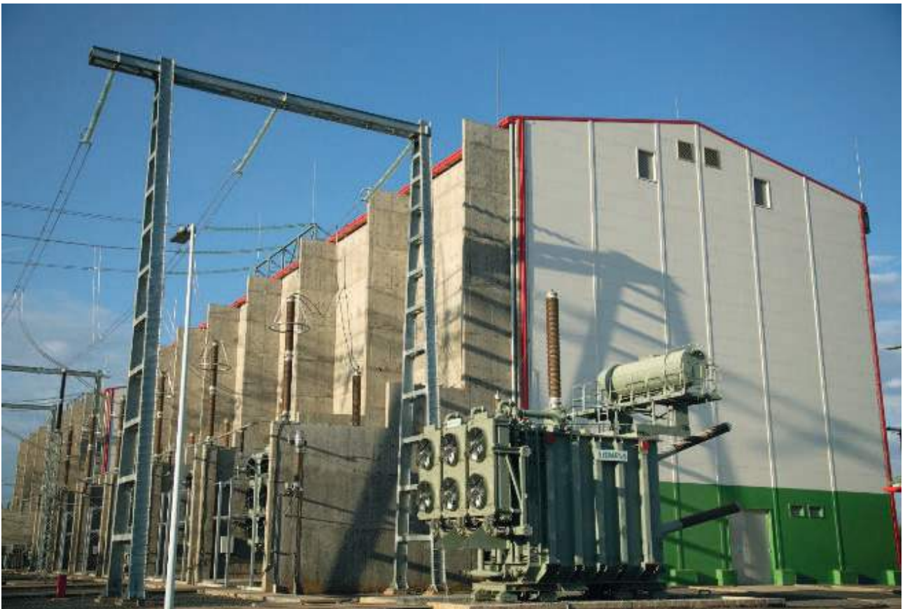
Converter Station for the 641km, 500kV Ethiopia-Kenya High Voltage Direct Current (HVDC) Transmission Line
