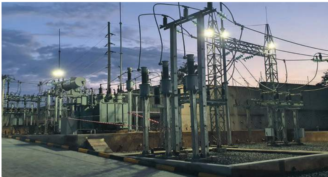
33/11kv, 7.5MVA Gatakaine Substation, Murang'a County
