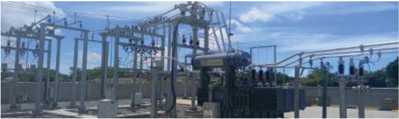
33/11 kv Sabaki Sub Station
