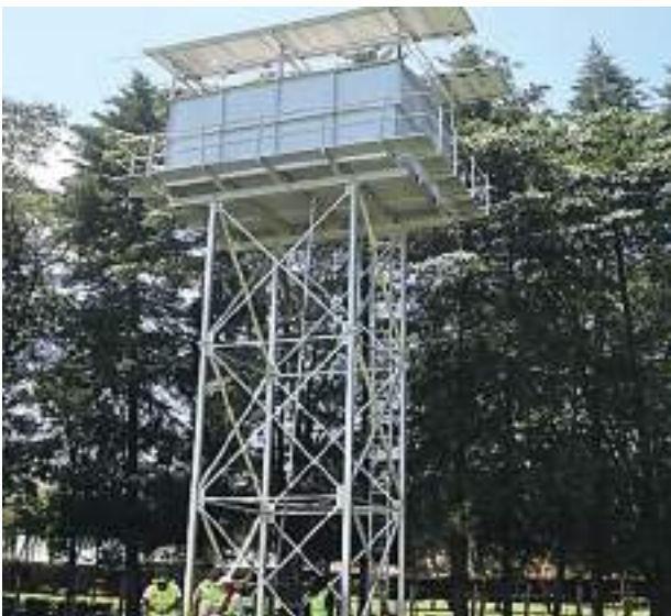
Exploratory borehole at Kakibei Primary in Kericho has been equipped with a water pump, a steel elevated tank of 24,000m 3 , and 16 high voltage solar panels.
