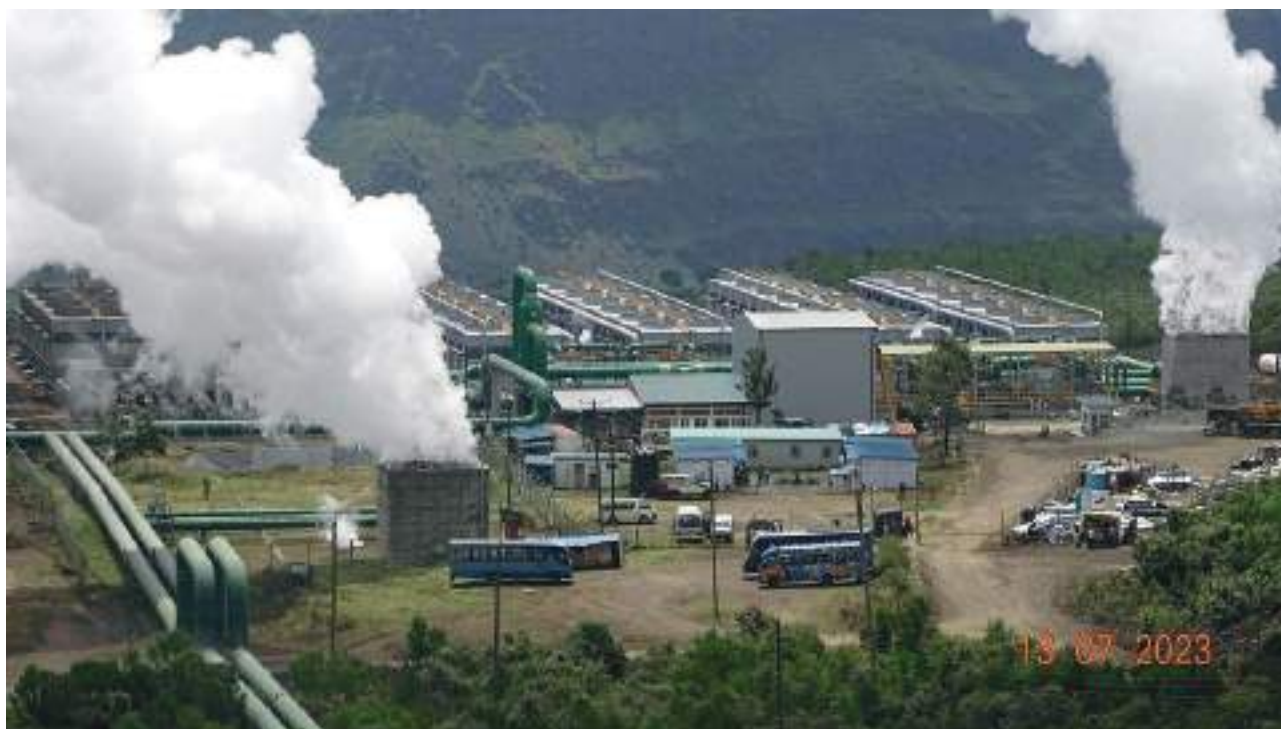
35MW Sosian Menengai Power Plant in Nakuru County
