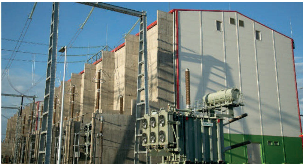
Converter Station for the 641km, 500kV Ethiopia-Kenya High Voltage Direct Current (HVDC) Transmission Line
