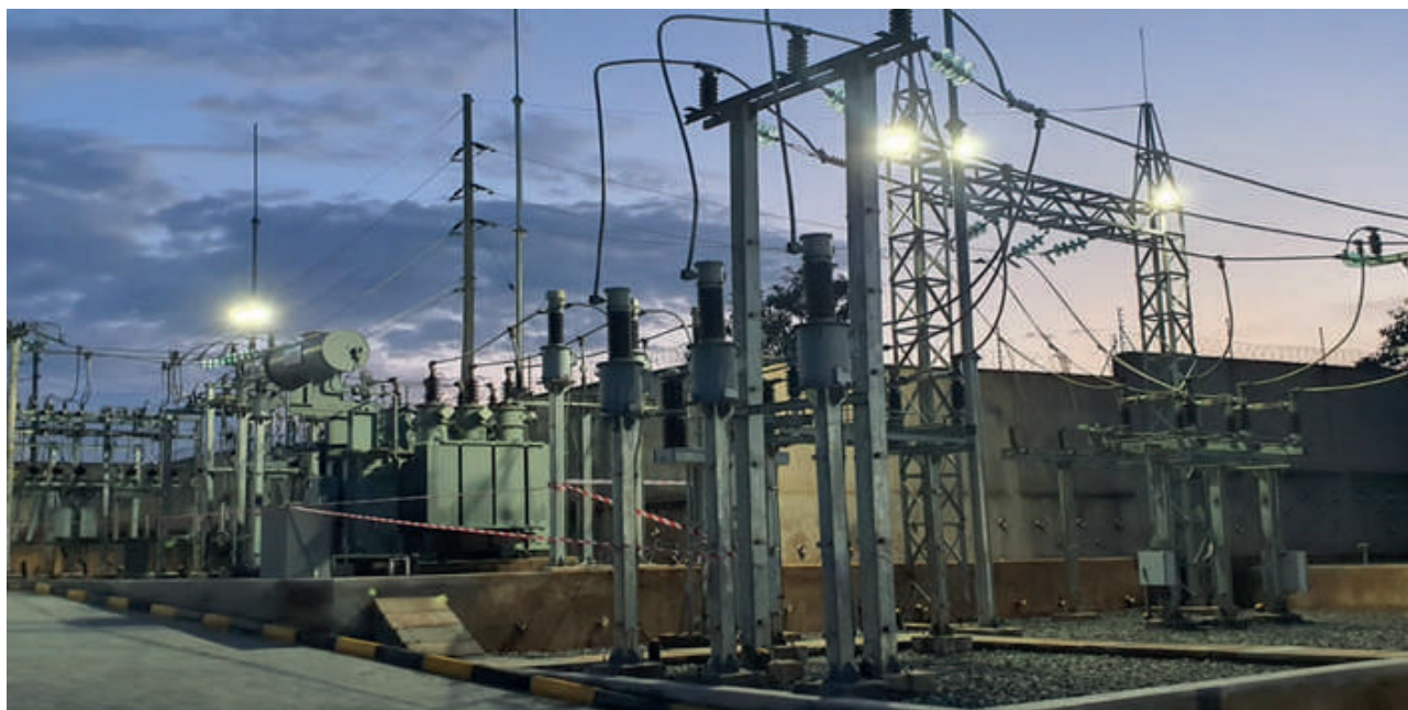
33/11kv, 7.5MVA Gatakaine Substation, Murang'a County
