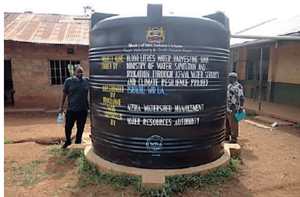
SCMP Implementation through construction of a Rainwater harvesting tank well installed at St Gerard Injira Primary School through Isiukhu WRUA.
