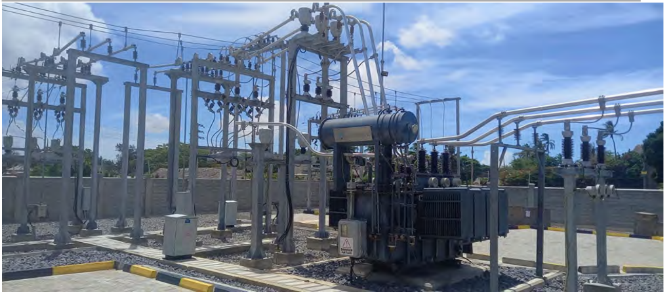
7.5MVA, 33/11kV Sabaki Sub-Station
